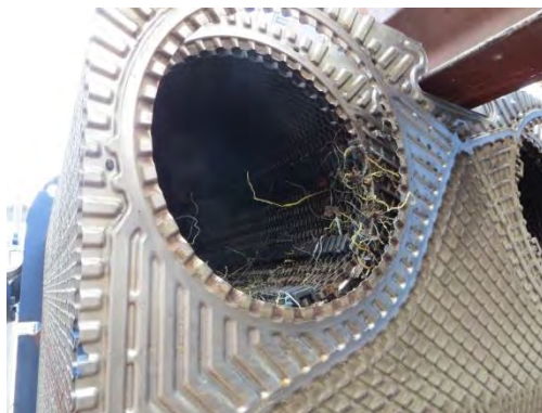
Dirt on inlet side
