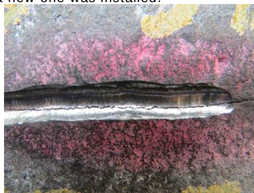
Crack close up after exposure grinding
