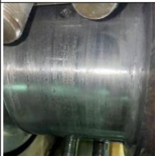
Main Journal from unit #1 as found. Its recommend to remove the complete crankshaft for engine frame housing evaluation.
